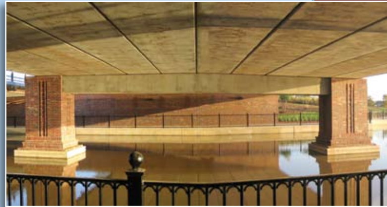
Side view of inverted-Tee bent cap, which enabled box beams to be supported by just two columns.
